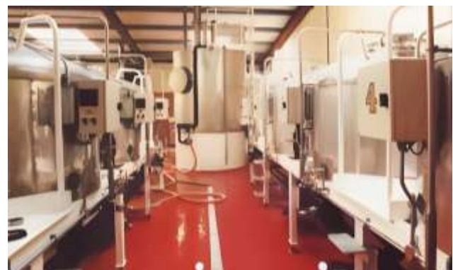
A complete RMDG installation at Leicester Clubs brewery in 1982.
