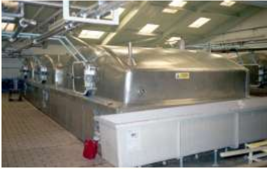
No3 fermenting room was installed at Cheltenham in 1963.
