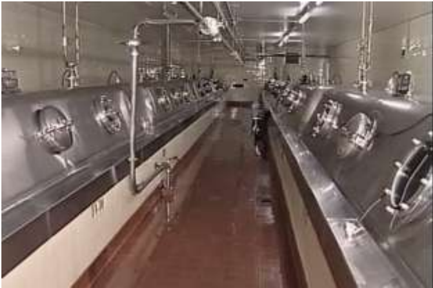
The fermenting room and (right) the conditioning tank corridor
