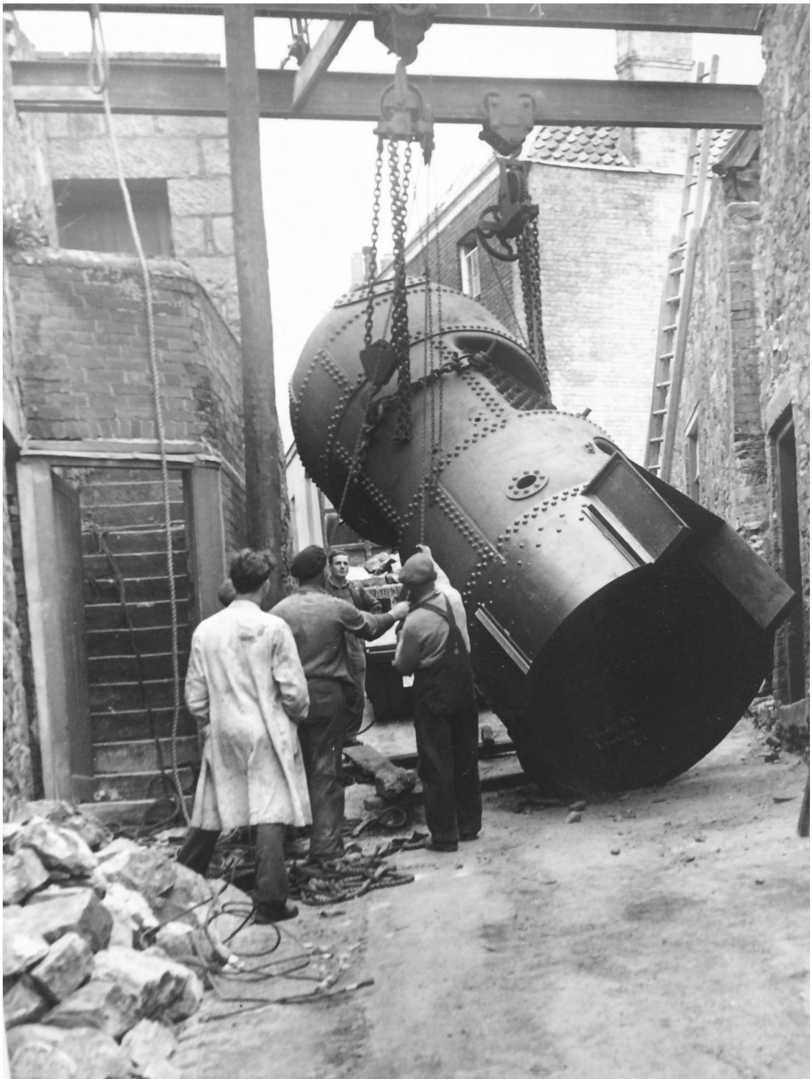
Figure 10. Replacing the boiler pre second world war.
