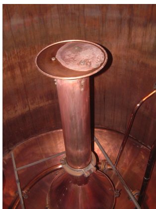
Figure 56. The calandria inside the copper at Arkells (2001).
