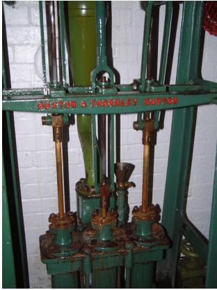
Figure 17. The power of steam at Hook Norton. Belt driven pumps.
