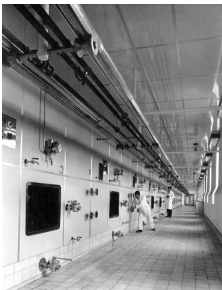
Figure 7. Redox tanks behind a posh fascia at Cape Hill, Birmingham (NBHT).
