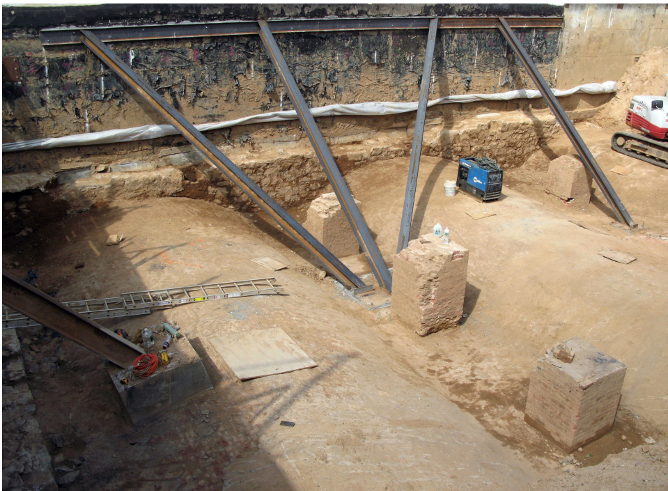
Figure 22. View over vaults 1 and 2 and piers 6, 7 and 8, to the west wall. Photo by Celia J. Bergoffen.
