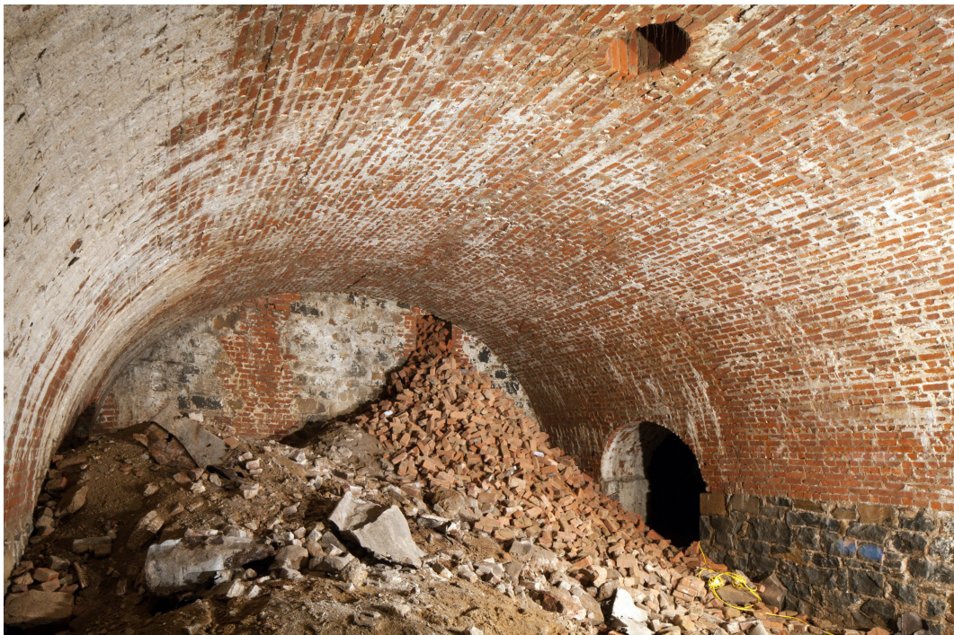
Figure 16. Vault 4: Upper ventilation shaft opening in the east wall (lower obscured by debris), opening in the roof of the vault, doorway to vault 3. Photo by Christopher D. Brazee.
