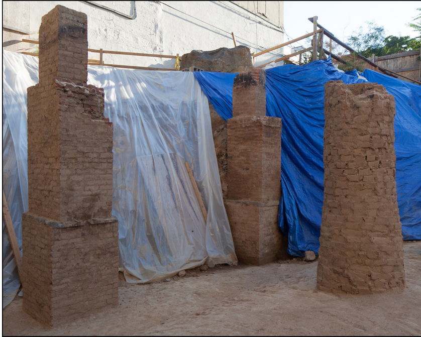
Figure 25. Chimney-shaped shaft on the top of vault 3 and piers 1 and 2. Photo by Christopher D. Brazee.
