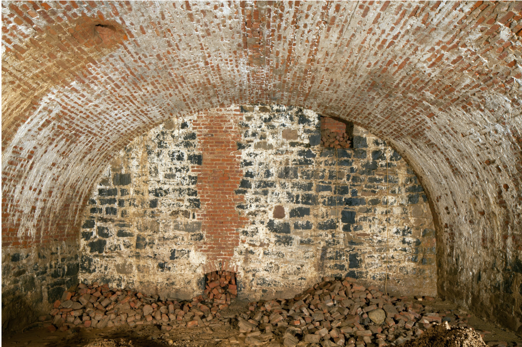
Figure 15. Vault 3: Ventilation shaft openings in the west wall, pipe (?) opening in the roof of the vault. Photo by Christopher D. Brazee.
