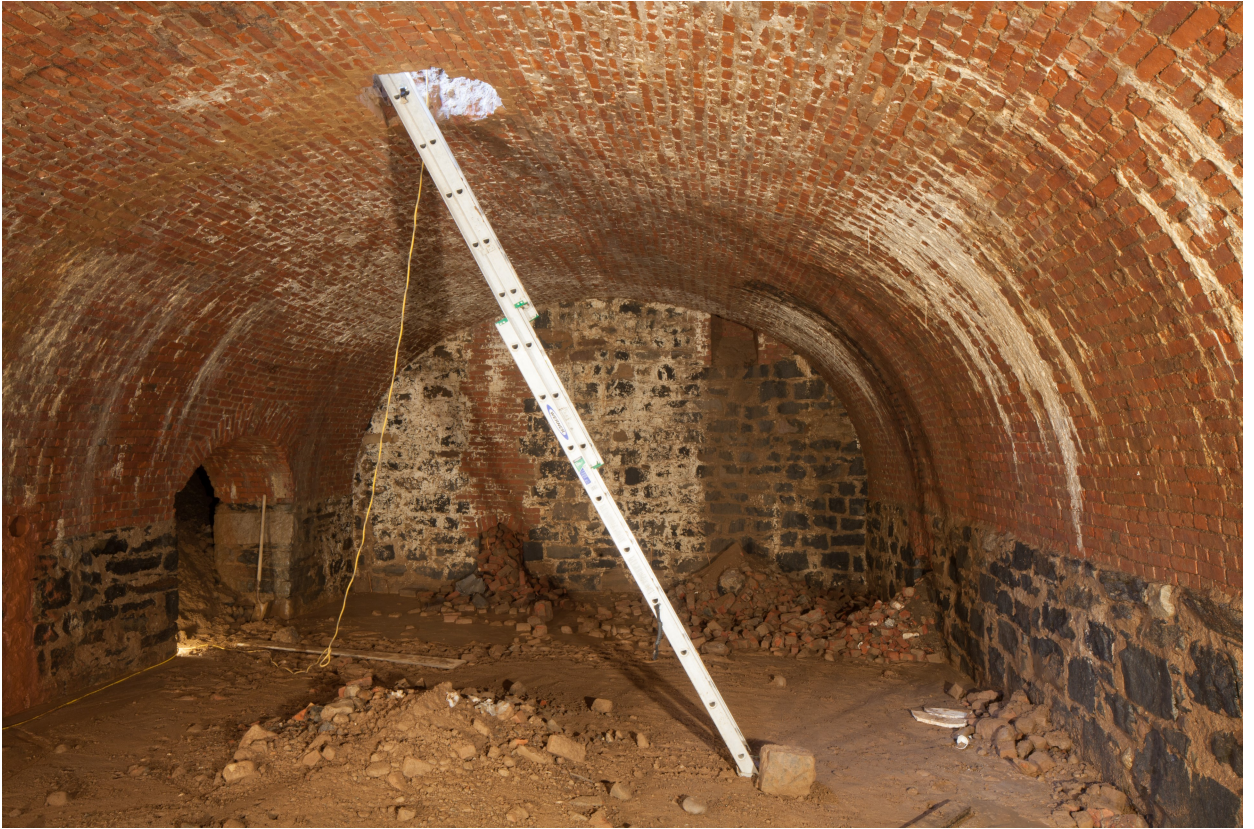
Figure 1. Vault 1: Access through the shaft opening in the roof of the vault, ventilation shaft openings in the east wall, doorway to vault 2. Photo by Christopher D. Brazee
