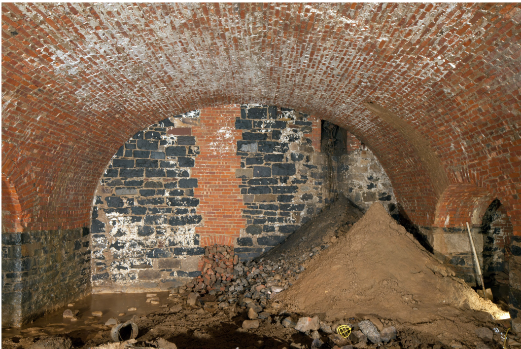
Figure 12. Vault 2: Ventilation shaft openings in the east wall, doorway to vaults 3. Photo by Christopher D. Brazee.
