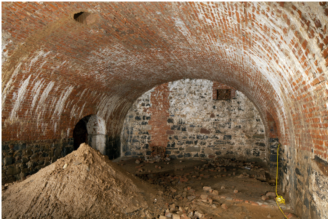
Figure 14. Vault 3: Ventilation shaft openings in the east wall, shaft opening in the roof of the vault, doorway to vault 4. Photo by Christopher D. Brazee.
