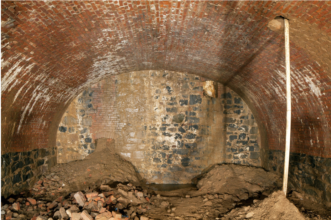
Figure 11. Vault 1: Ventilation shaft openings in the west wall, pipe (?) opening in the roof of the vault. Photo by Christopher D. Brazee.
