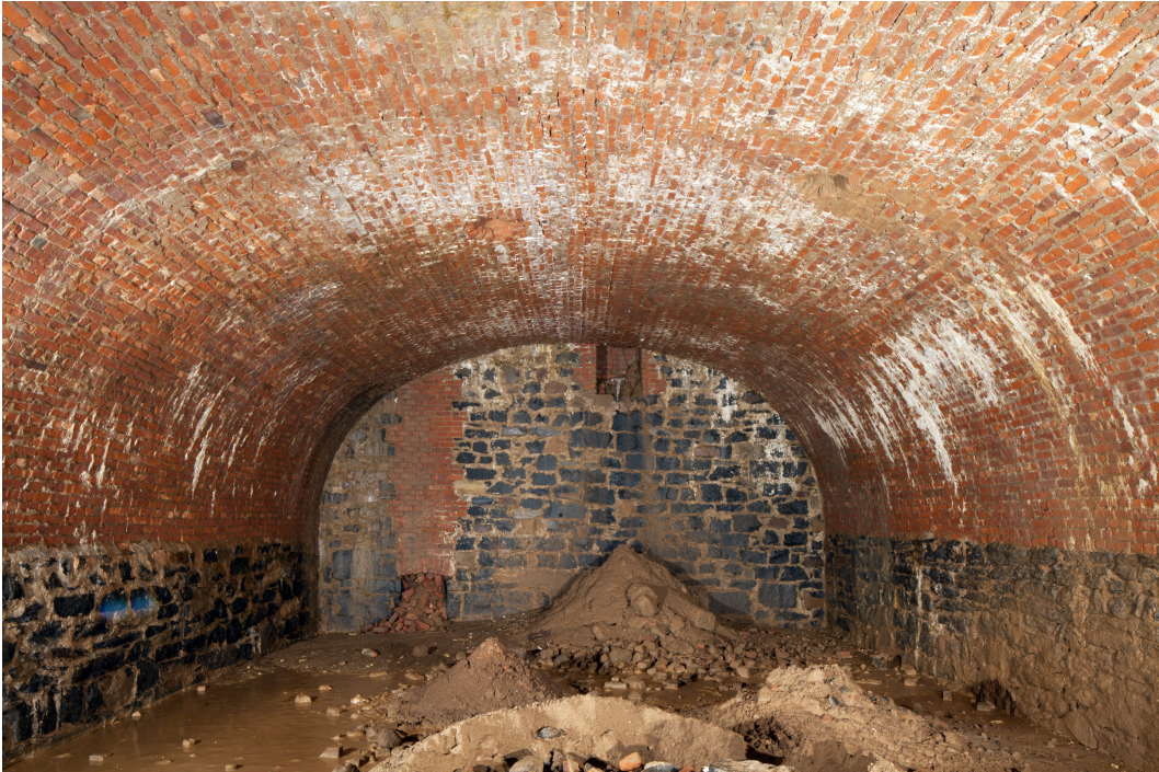
Figure 13. Vault 2: Ventilation shaft openings in the west wall. Photo by Christopher D. Brazee.
