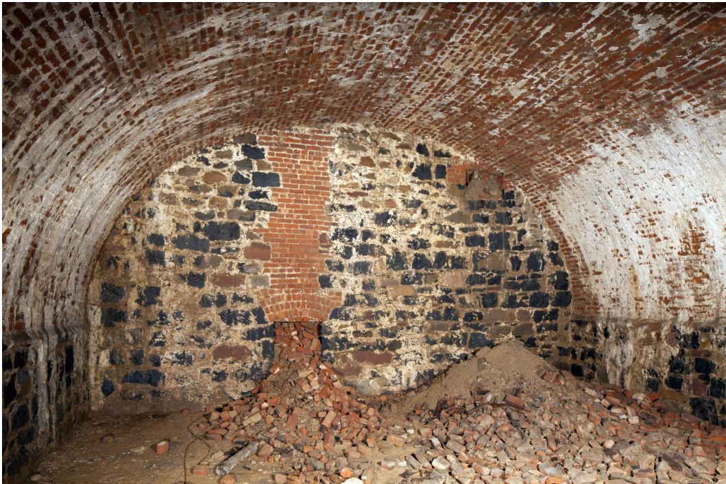
Figure 17. Vault 4: Ventilation shaft openings in the west wall. Photo by Christopher D. Brazee.
