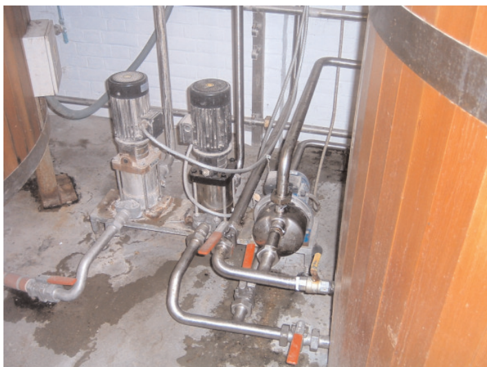
Figure 5. Pumps and filters.
