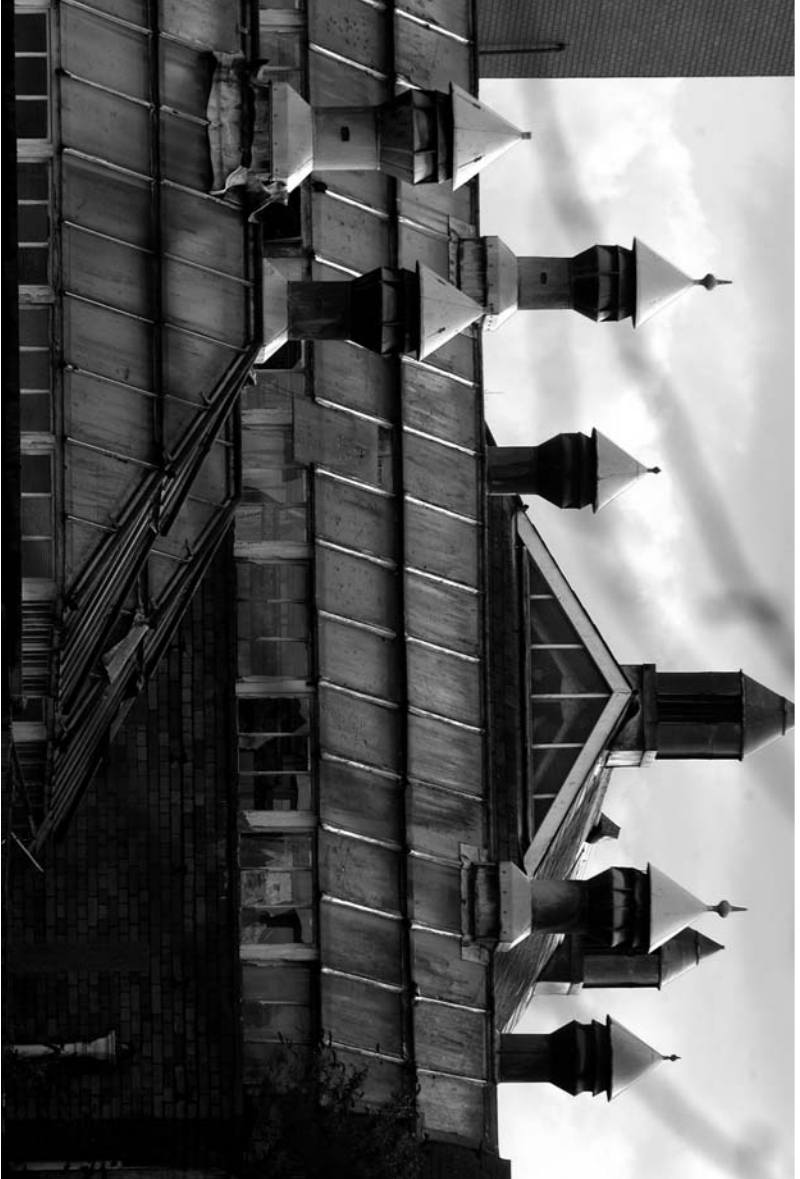
Figure 1. The view is taken from what is now Castle Park, across the River Avon. One of the chimneys in the foreground was nearly lost to copper thieves. (All photographs by Stephen Morris).
